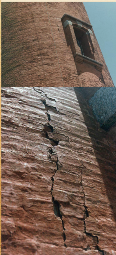
CRACKS IN THE PONCE (MOSQUITO) INLET LIGHTHOUSE TOWER
