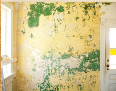
PLASTER DAMAGE ON THE SOUTH WALL OF LIVING ROOM.
