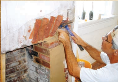
ED MILANO WORKS ON THE LIVING ROOM FIREPLACE REPAIR IN THE SECOND ASSISTANT KEEPER'S DWELLING.
