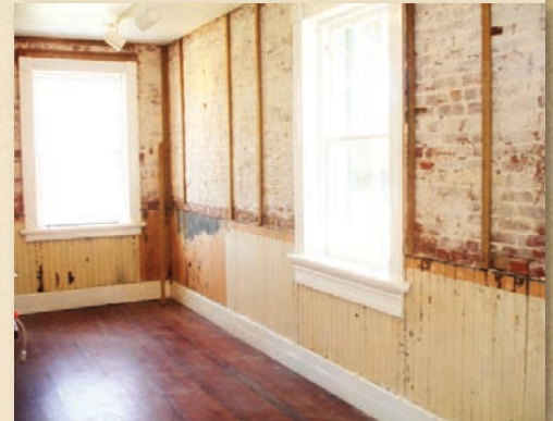
ORIGINAL BEADBOARD WAINSCOTING WAS HIDDEN UNTIL PANELING WAS REMOVED IN THE KITCHEN AREA.
